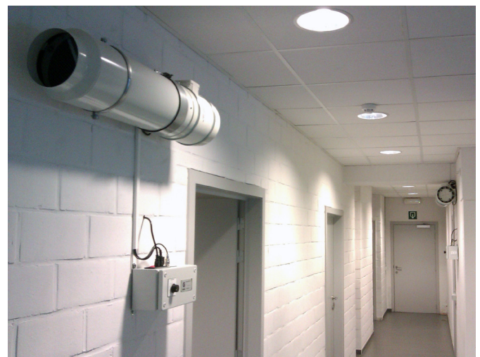
A corridor installation where several Genano® Tube XS air purifiers are used together for optimal results.
